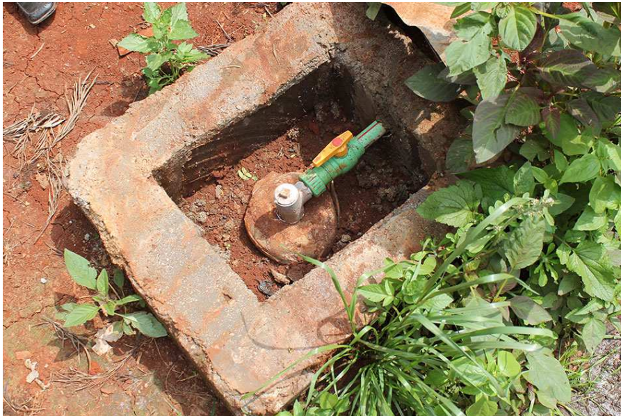
Figure 2: Biogas outlet from which biogas is fed into the household, ready for use
